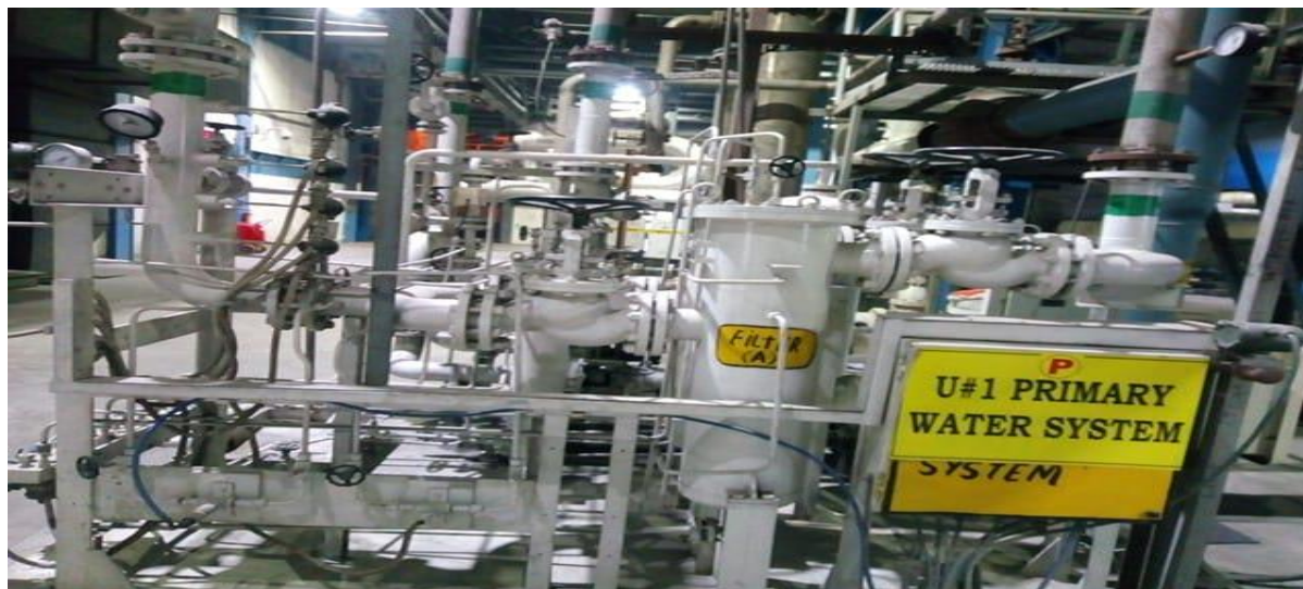
Fig-5: Photograph of Primary Water System in 500MW unit
